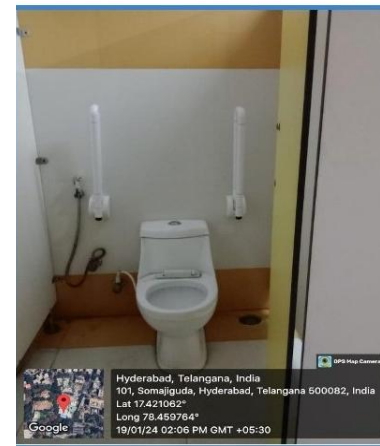
DISABLE - FRIENDLY WASHROOM
